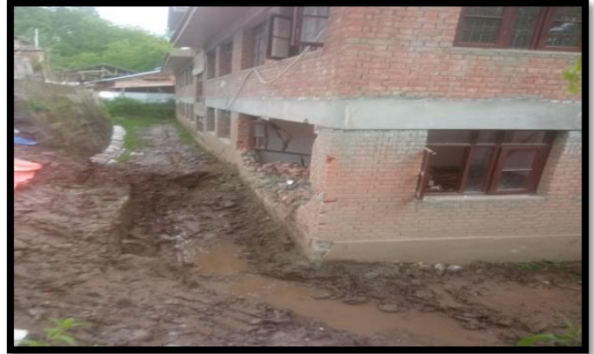
Damaged Portion of the Building
